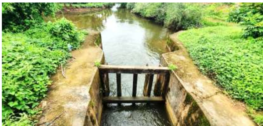
a sluice gate
